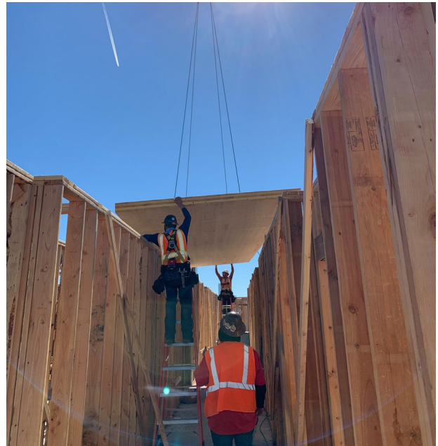
Installation of Kattera CLT at Cirrus, a 292-unit multifamily mid-rise building in Denver, CO. Five- and seven-ply CLT panels will be used for five stories of exposed ceilings.
