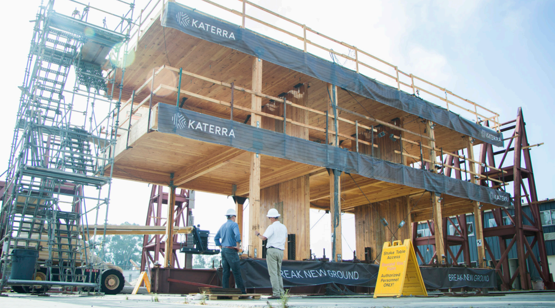
In 2017, a two-story seismic shake table test validated the performance of Katterra's patented CLT shear wall system.
